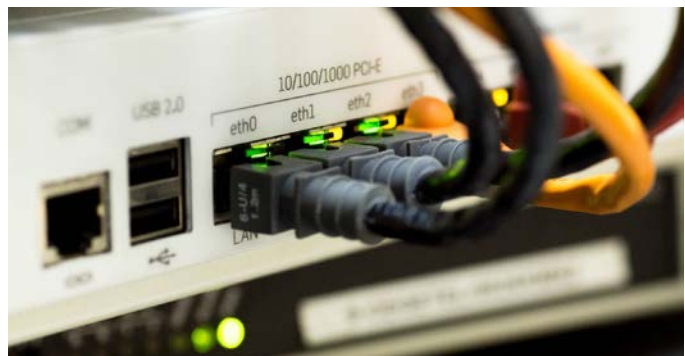
Figure 10.12: Cables connected to a network switch
